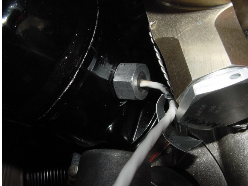
Figure 21-17 Magneto Tach Sensor Installed
