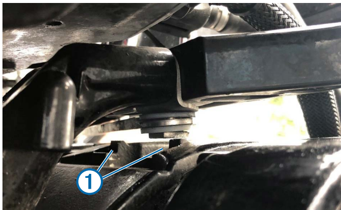
Side View of Reactor 40 Kicker Steering Actuator Bracket
